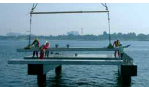
The erection team has gone offshore to erect heavy columns, beams and hollowcore slabs on a foundation.
