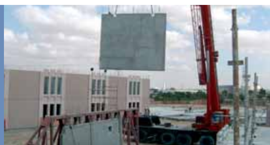
Another of the total of 4,500 m 2 wall panels is lifted to its final position on American School in Abu Dhabi.
